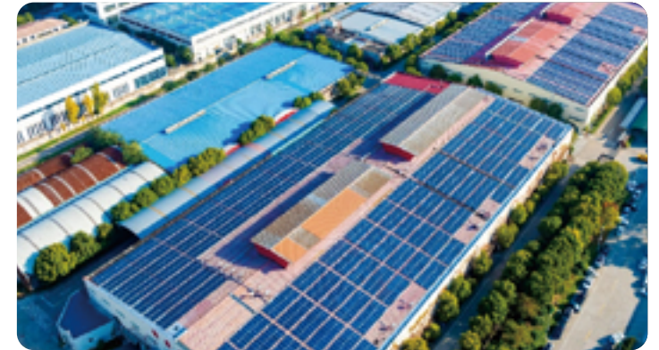
Distributed Rooftop Photovoltaic Power Stations
