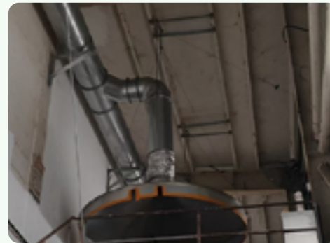
Waste gas collection devices were added to the wastewater pretreatment section of the dipping workshop to reduce fugitive waste gas emissions.
