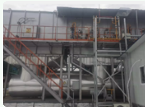
A new RTO waste gas treatment device was built in the dipping workshop of Haiyang Polyamide
