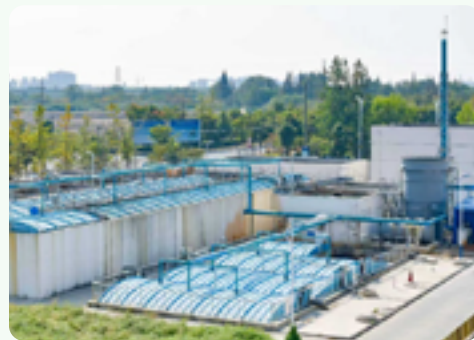
Wastewater Treatment Facilities of Haiyang Polyamide
