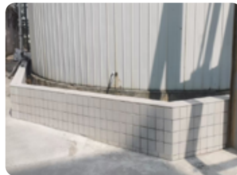
Cofferdams were added to the tank farm of Haiyang Polyamide to reduce the risk of pollution caused by raw material leakage.
